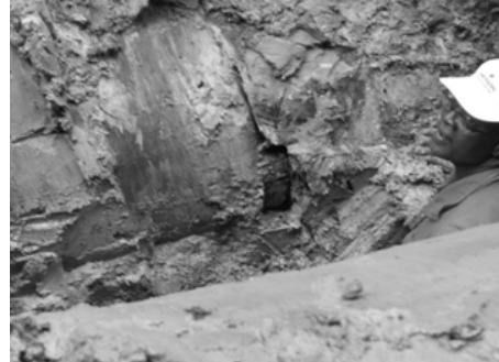
Fig. 12. Defect found from data in Fig. 11
